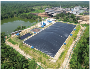
GLT Maju 1.5MW Biogas Power Plant
